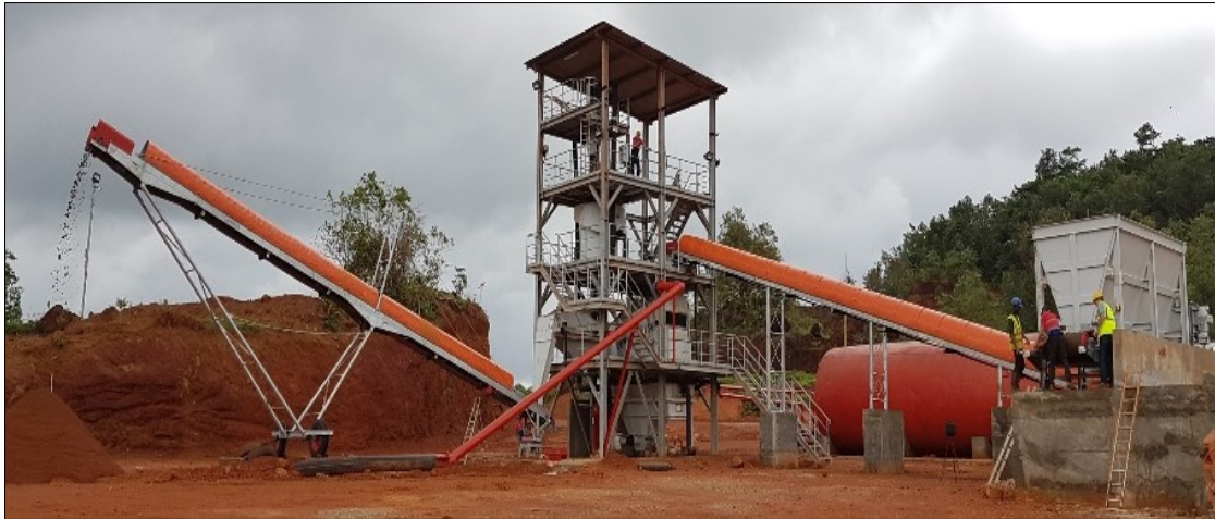
Figure 17. Processing plant stock tailings. The box feeder on the right side will be filled by wheel loader with the bulky stock tailings material and the same vertical process arrangement as the fresh tailings.
